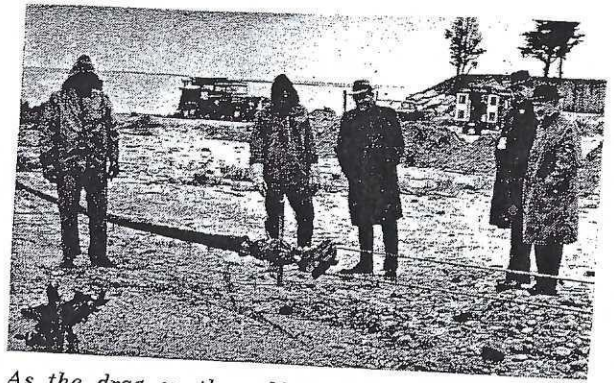
As the drag on the cable has become quite heavy the direct pull with the steel rope has been changed by running the steel rope through a snatch block called a "whip." Making this change are Art Frost and "Babe" Burlingame. Observing are Outs. Plt. Engs. Frank Ormon and Ted Taylor, who designed and engineered the job, also Manager Ed Cross.
